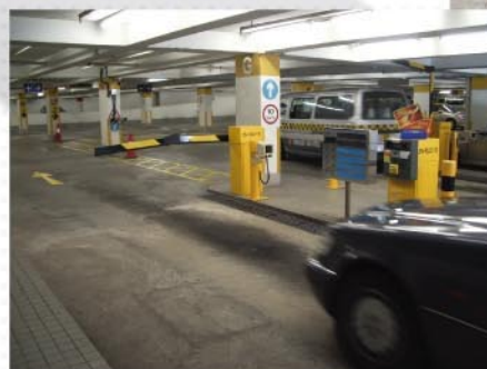
VECON-JANITOR at Indoor Car Park
